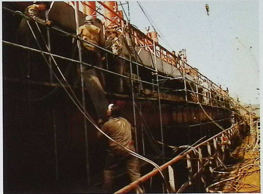
▲ Extensive wingtank repairs were executed on m.t. „Bow Cedar” – Rederiet Odffjell A.S., Bergen, Norway. For this purpose a strake of about 80 metres of hull plate had to be removed on both sides.
